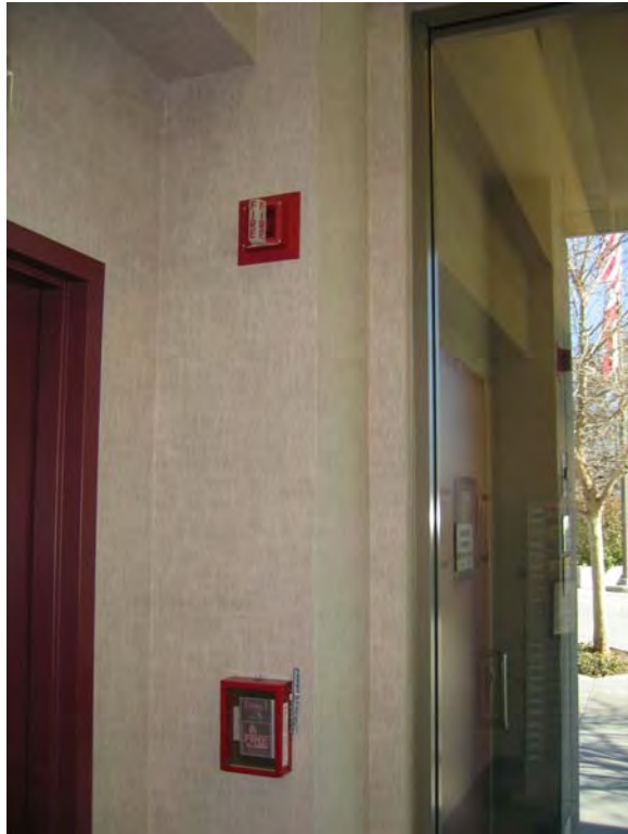
Student Services Strobe and Pull Station
