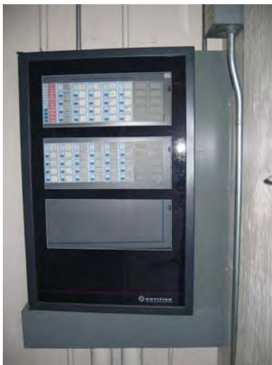
Tech Building Fire Alarm Control Panel
