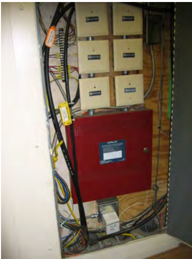
Fire Alarm Subpanel "FAD"
