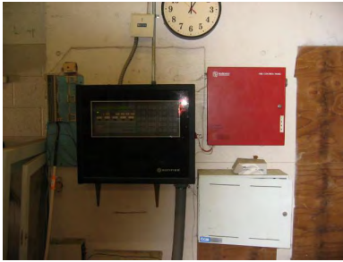
Fire Alarm Main Panel (Mech Bldg 1)
