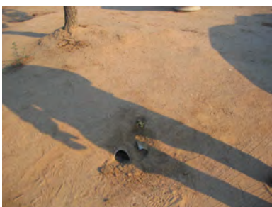
Two 4 inch conduit from HH #BB South side
