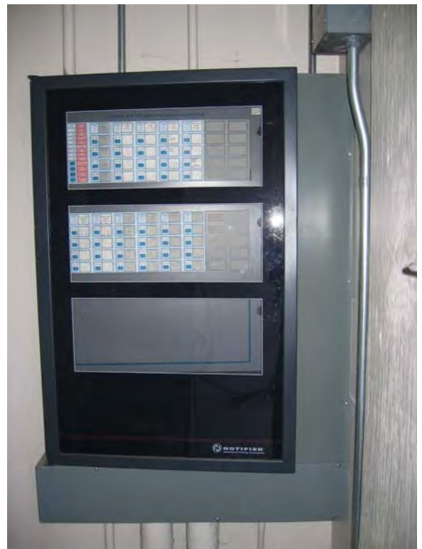
Tech Building Fire Alarm Control Panel
