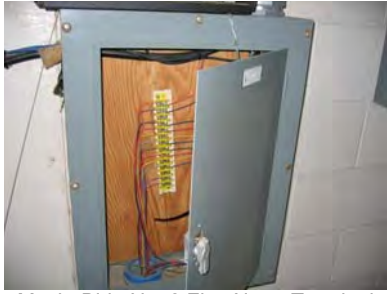
Mech. Bldg No. 2 Fire Alarm Terminal Cabinet
