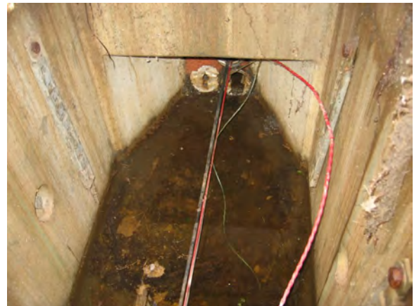
Fire Alarm Pullbox "PB-1"
