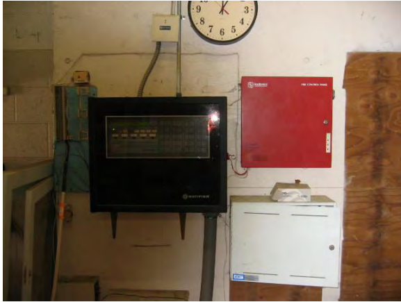
Fire Alarm Main Panel (Mech Bldg No.1)
