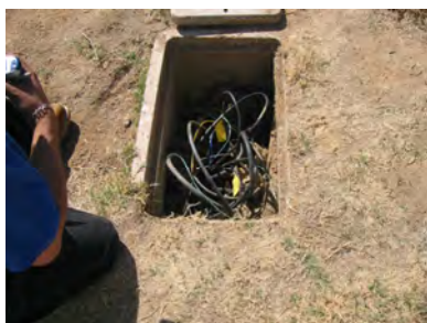
HH #CC Copper and fiber optic cables
