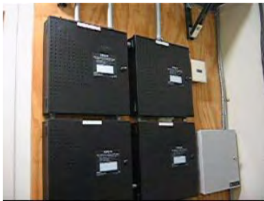
Humanities Building Fire Alarm Module
