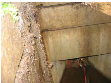
Fire Alarm Pullbox "PB-1"
