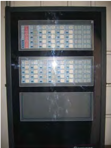
Library Fire Alarm Control Panel
