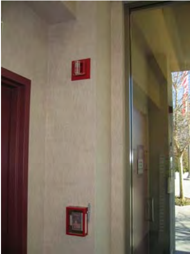
Student Services Strobe and Pull Station
