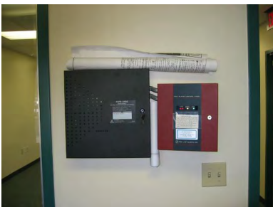
Stand-Alone Fire Alarm System
