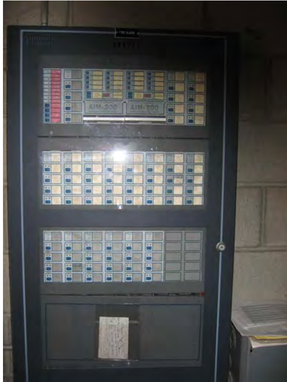
Central Plant Fire Alarm Main Panel
