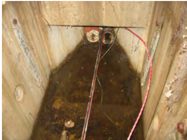
Fire Alarm Pullbox "PB-1"
