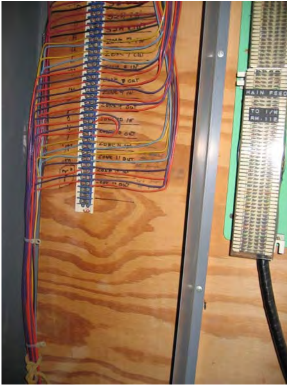
Science Tech Fire Alarm Terminal Cabinet
