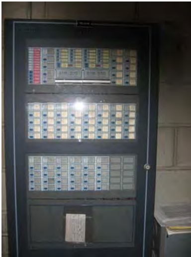
Central Plant Fire Alarm Main Panel
