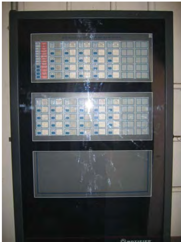
Library Fire Alarm Control Panel
