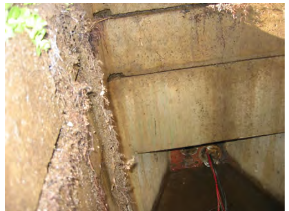
Fire Alarm Pullbox "PB-1"
