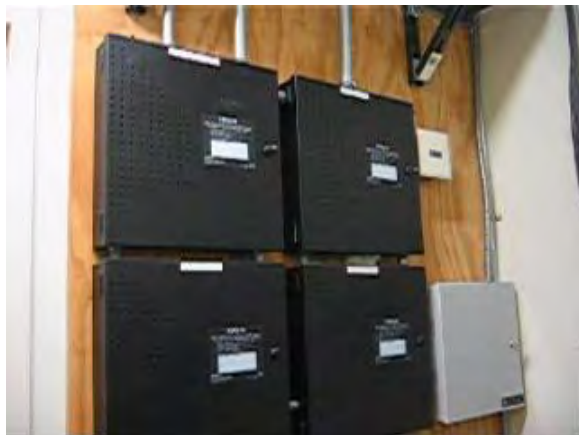
Humanities Building Fire Alarm Module
