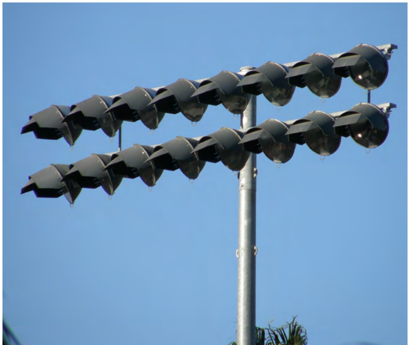
Sports lighting : Horizontal array with glare shield
