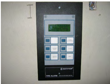
Fire Alarm Remote Annunciator "FAA"
