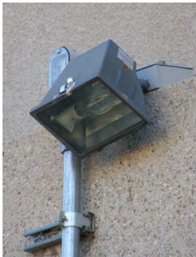
Roof mounted and wall mounted flood lighting fixtures
