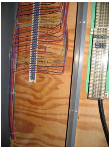
Science Tech Fire Alarm Terminal Cabinet
