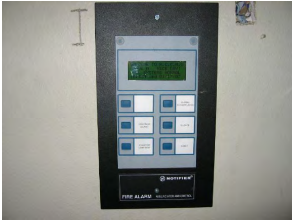
Fire Alarm Remote Annunciator "FAA" (Warehouse)
