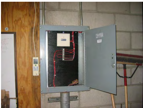
Fire Alarm Terminal Cabinet (Mech. Bldg. No.2)
