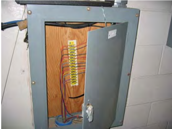
Mech. Bldg No. 2 Fire Alarm Terminal Cabinet
