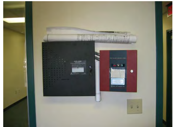
Stand-Alone Fire Alarm System (President's Office)
