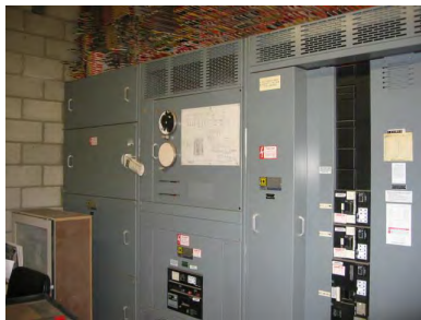
Main Switchboard "MSB2"
