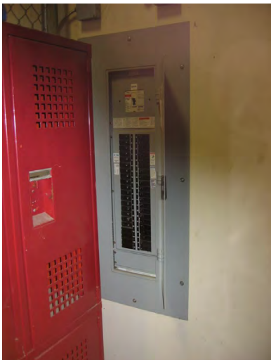
Warehouse Panel "WP" (South)
