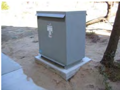
Multipurpose Bldg Transformer "TH"
