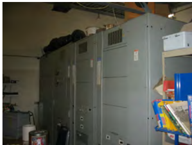
Main Switchboard "MSB"
