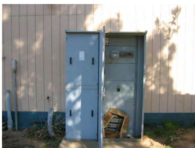
Old Main Switchboard "MS" (South)
