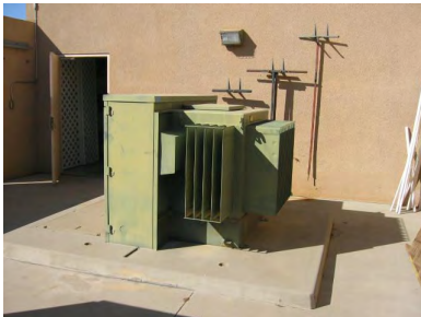
SCE 750 kVA Transformer Mech Bldg 1
