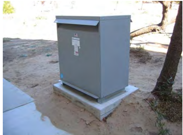
Multipurpose Bldg Transformer "TH"
