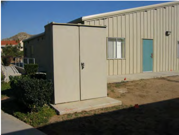
Main Switchboard "MSF" (South)
