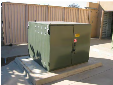
SCE Capacitor Bank Mech Bldg 1
