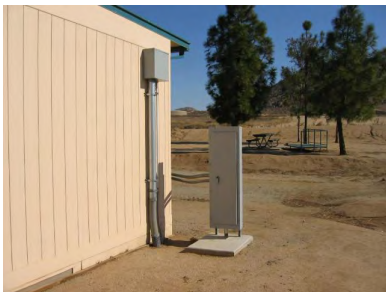
Power Panel "PP" (South)
