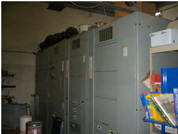
Main Switchboard "MSB"
