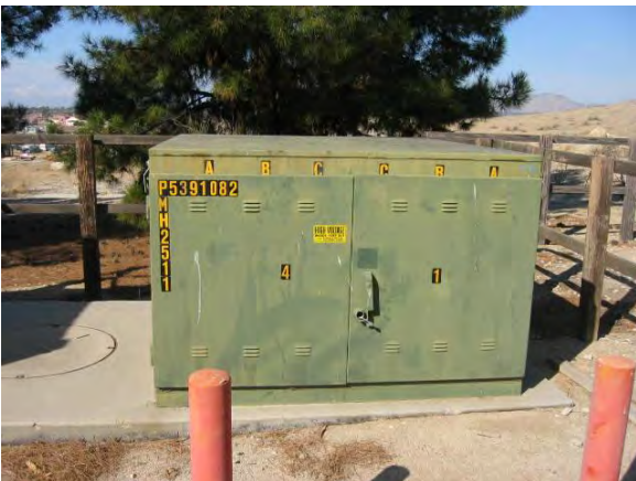
SCE Pullbox and Capacitor Bank
