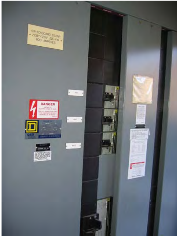
LV Switchboard DSBNP
