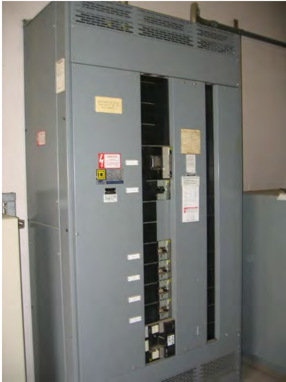
Library 800 Amp Switchboard
