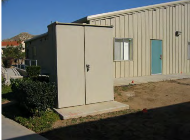
Main Switchboard "MSF" (South)
