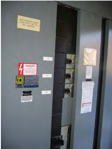
LV Switchboard DSBNP
