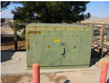
SCE Pullbox and Capacitor Bank
