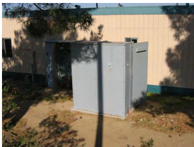
Main Switchboard "MSB" (South)
