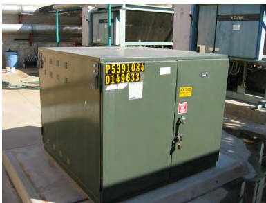
SCE Capacitor Bank Mech Bldg 1
