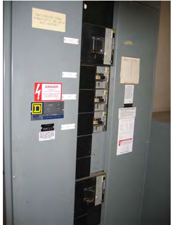
LV Switchboard DSBNL
