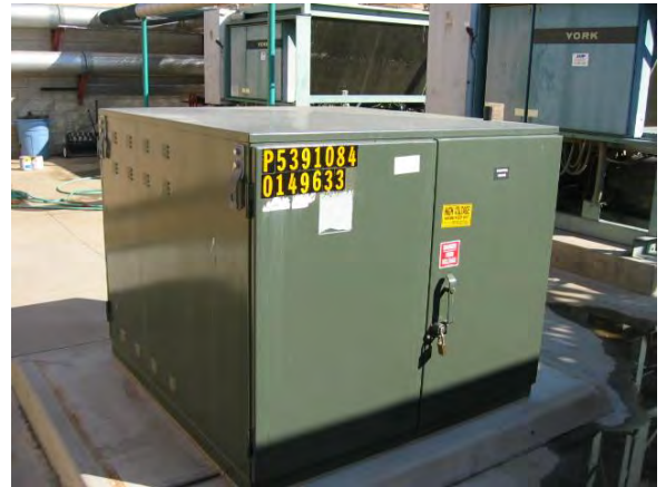
SCE Capacitor Bank Mech Bldg 1
