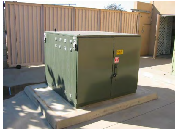
SCE Capacitor Bank Mech Bldg 1
