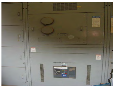
Main Switchboard "MSB"
