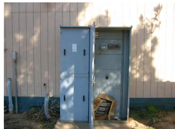
Old Main Switchboard "MS" (South)
