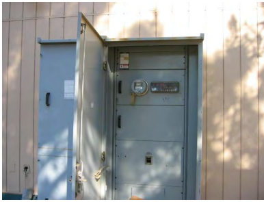
Old Main Switchboard "MS" (South)
