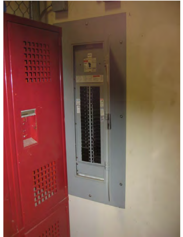
Warehouse Panel "WP" (South)
