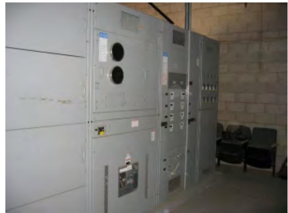
LV Main Switchboard (Facilities 1)
