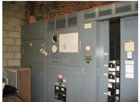
Main Switchboard "MSB2"
