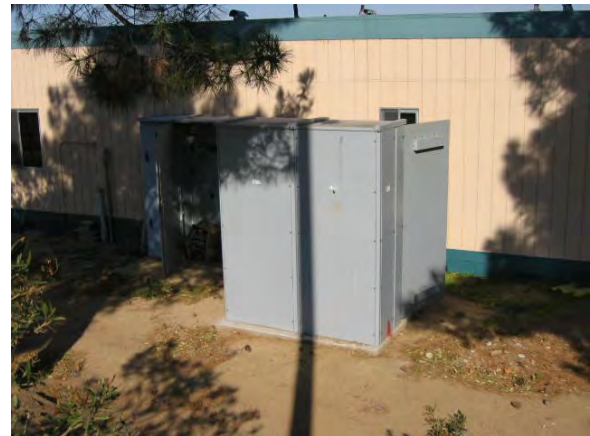
Main Switchboard "MSB" (South)
