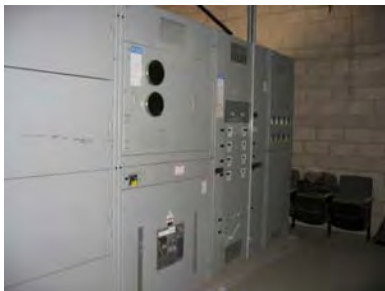
LV Main Switchboard (Facilities 1)
