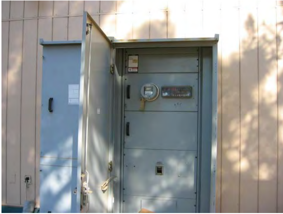
Old Main Switchboard "MS" (South)
