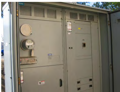
Main Switchboard "MSB" (South)
