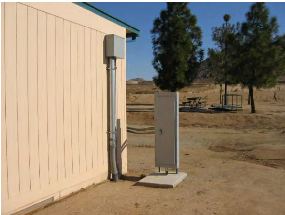
Power Panel "PP" (South)
