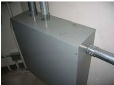
Multipurpose Bldg Pullbox
