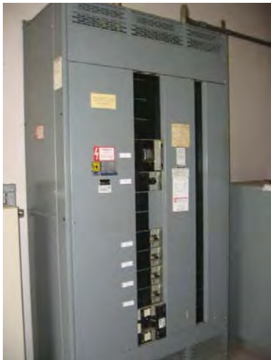
Library 800A Switchboard
