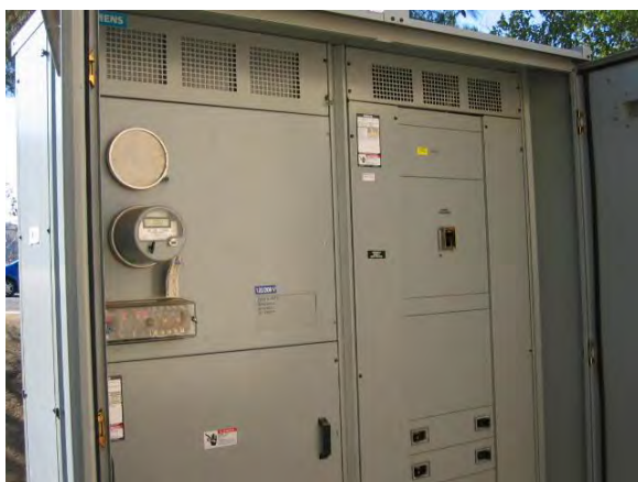
Main Switchboard "MSB" (South)
