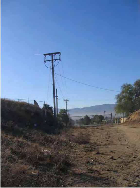
SCE Power Pole on Mountain Ave.
