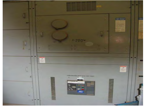
Main Switchboard "MSB"
