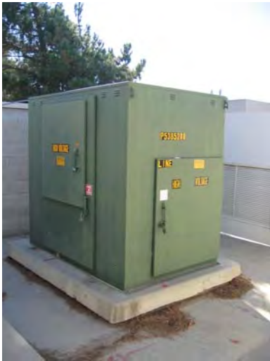
SCE HV Switch &amp; Meter Enclosure
