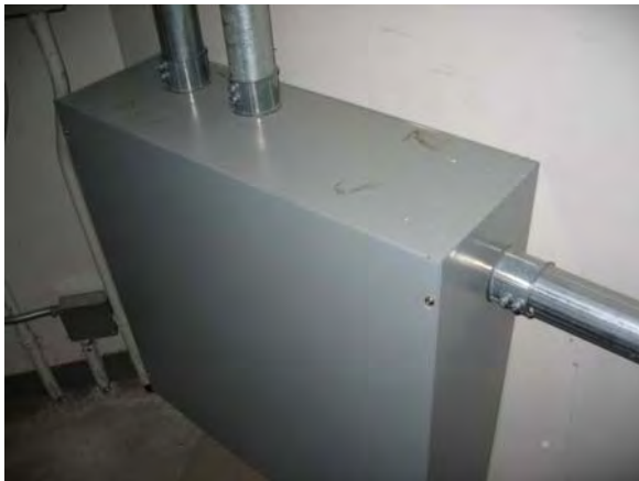
Multipurpose Bldg Pullbox
