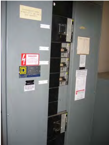
LV Switchboard DSBNL
