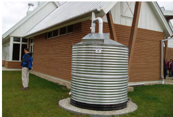
Rain Storage Tank/Cistern
