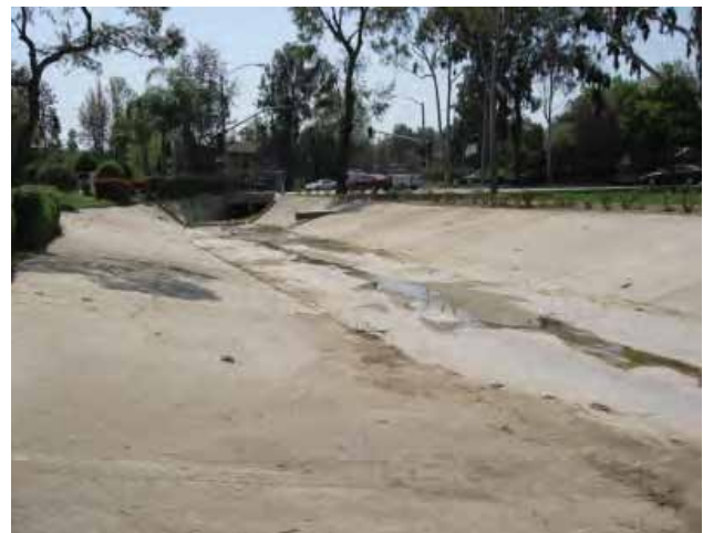
Drainage channel through campus is part of a regional watershed system
