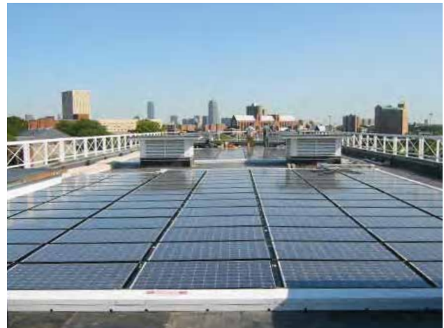
Rooftop photovoltaic array at Harvard University
