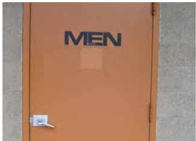
Inconsistent and non-ADA compliant restroom identity
