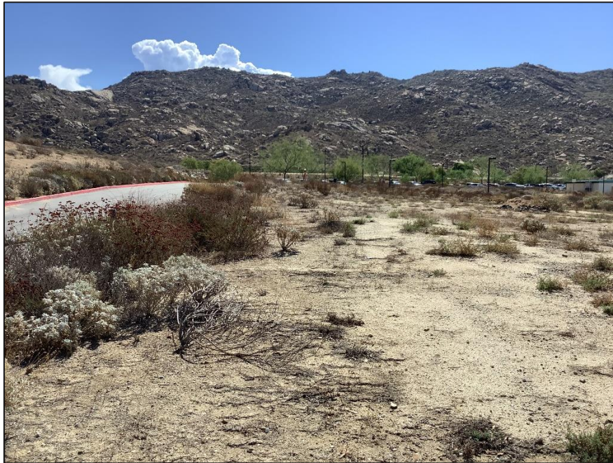
Image 12. View of New 12 kV Underground Line where it connects to the Existing 12 kV Underground Line Work Area, looking east/northeast (IMG_0688)
