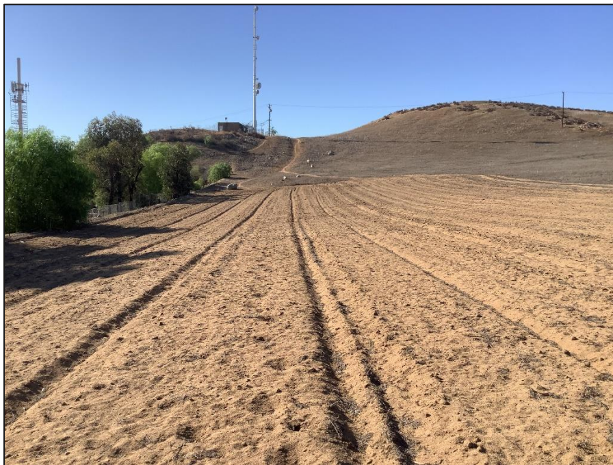
Image 6. View of area south of PV Solar Array Work Area, looking south (IMG_0670)
