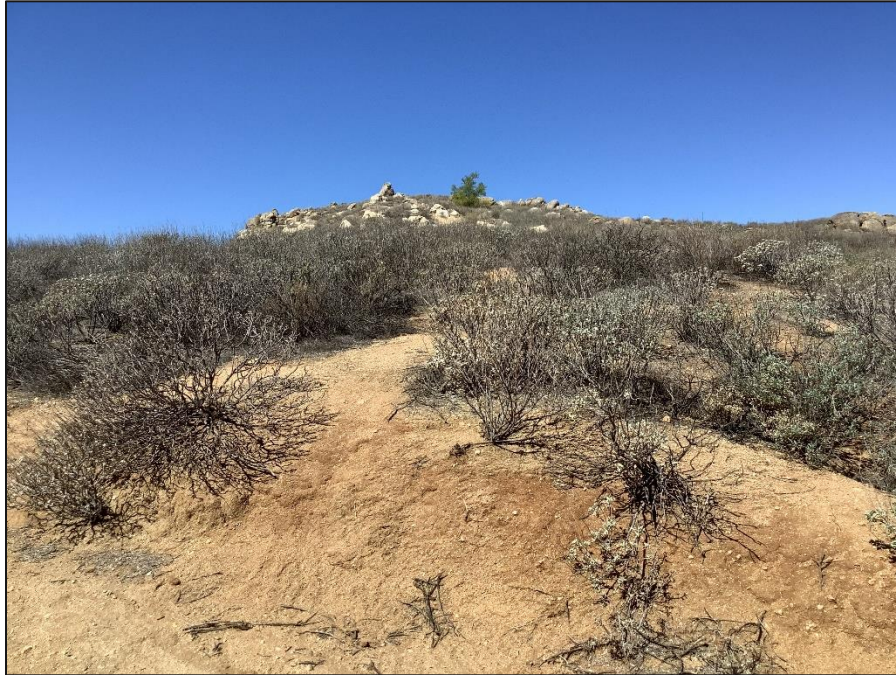
Image 14. View of the New 12 kV Underground Line Work Area, looking north towards the Mount Russell Hills (IMG-0702)
