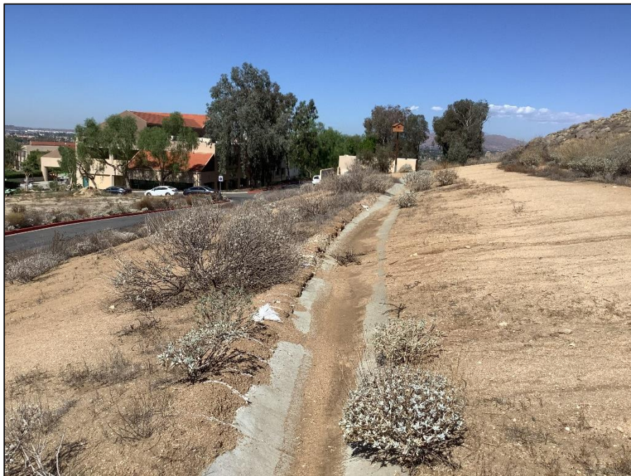
Image 13. View of concrete-lined water diversion channel within the New 12 kV Underground Line Work Area, looking west (IMG-0698)
