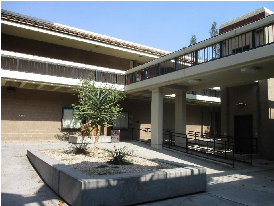
Figure 7. Life Science, portion of east elevation and cafeteria elevated walkway, looking northwest (IMG_5190)
