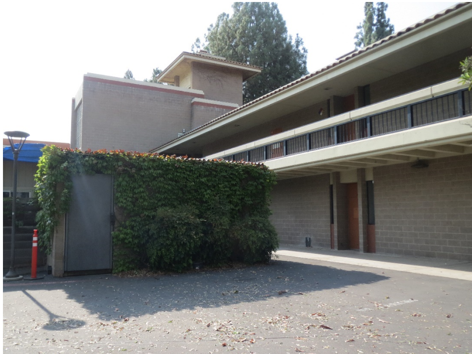
Figure 38. Physical Science Building, portion of North elevation, clocktower behind, looking southeast (IMG_4528)
