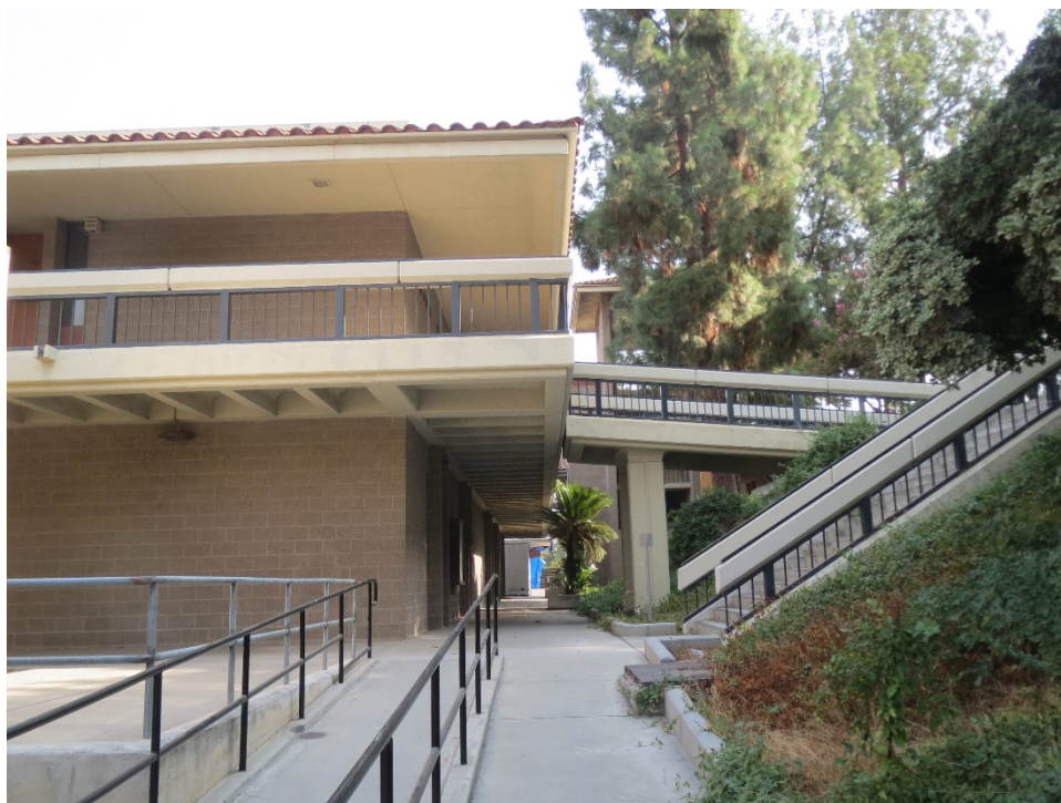
Figure 33. Physical Science Building, portion of South elevation, detail of ramp and stair looking north (IMG_4500)
