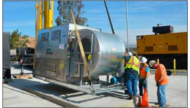
Fuel Cell Project at Norco College
