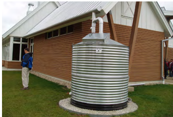
Rain Storage Tank/Cistern
